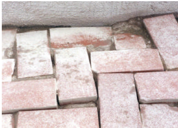
Loss of interlock due to sand loss through weep holes, Ohio
