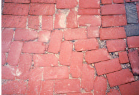
Edge Chippage, Ohio August 2000 Figure 7
