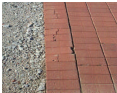
Cracking along edge, South Carolina Area #1 March 2001 Figure 6
