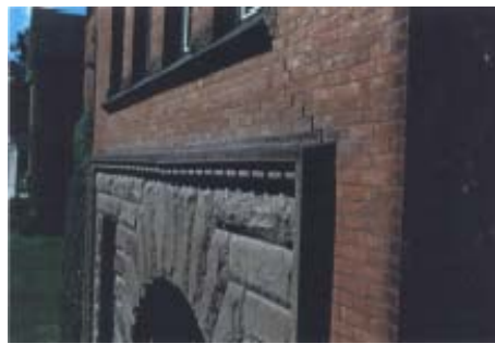
Figure 2. Settled coping stone and deformed brickwork.
