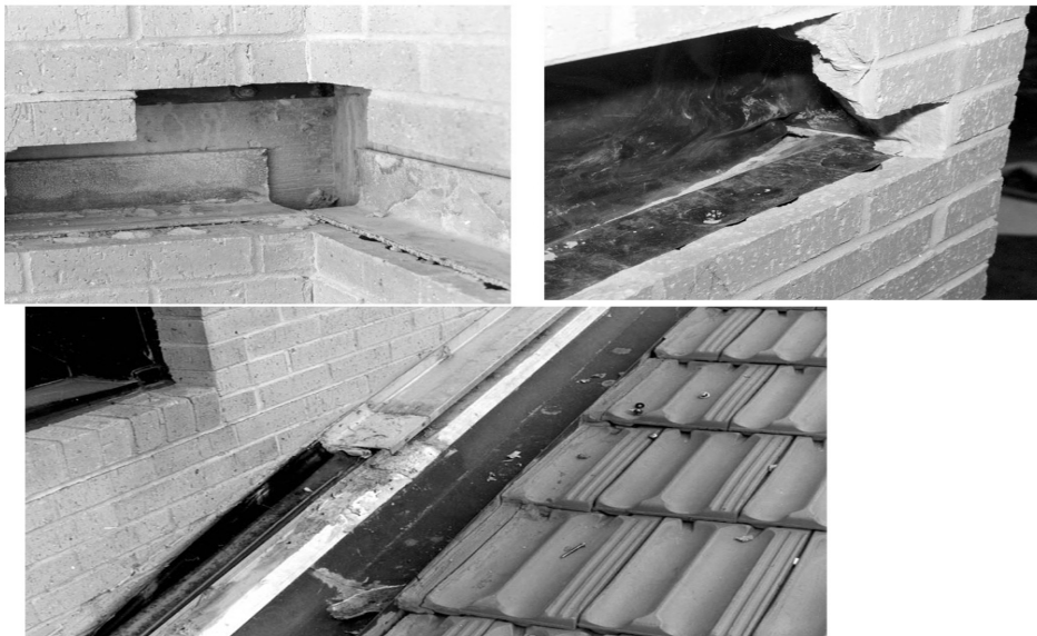
Figure 3. Thru-wall flashing is missing at shaft angles (top left) and roof to rising wall intersections (bottom). Where flashing is present, it is unsupported and unsealed at joints.
