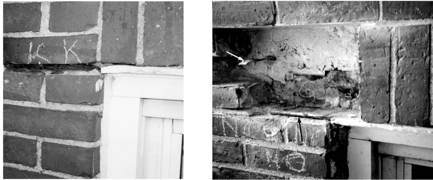
Figure 2. Copper lintel flashing lacks end dams to protect embedded steel, which has rusted and expanded, spalling mortar from the brick joint.
