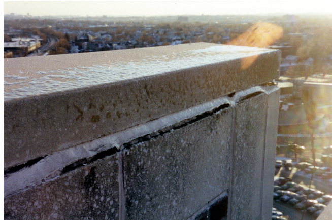
Fig. 4. Flashing beneath these coping blocks terminated behind sealant. The resulting water ingress rusted reinforcing steel beneath the blocks and heaved them upward.
