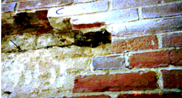
Figure 1. Asphalt-impregnated fabric through-wall flashing has decayed; all that remains is black residue in the bed joint.
