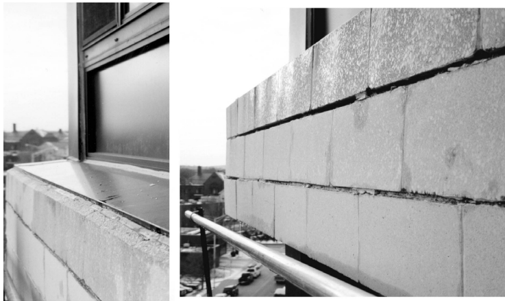
Fig. 5. Significant damage has been caused by the termination of sill flashing above the concrete block, and by failure to extend flashing over the face of the block. These defects directed water into the masonry.
