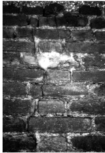
Figure 4. Thin cracks on the wall
