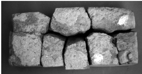
Figure 6. Cracked brick sampled inside the damaged wall
