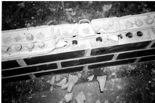
Figure 9- Photograph of a failed specimen showing mortar split due to presence of joint reinforcement wire
