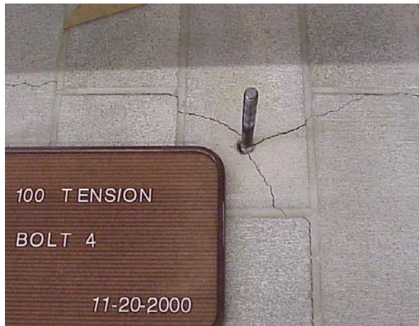
Figure (4): Radial Cracking
