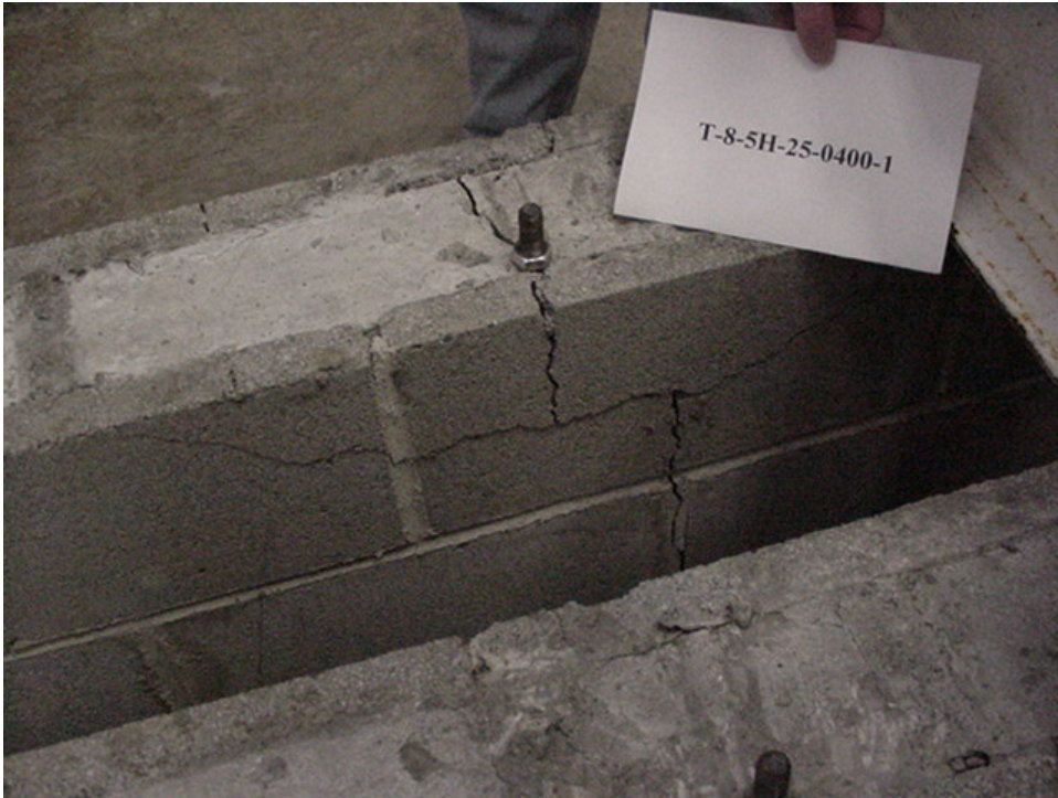
Figure 6. Failed Specimen T-8-5H-25-0400-1
