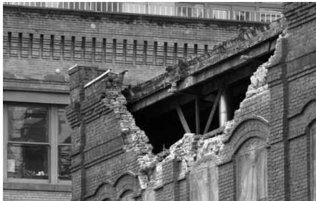
Figure 2. Out-of-plane wall failure in the 2001 Nisqually Earthquake.
