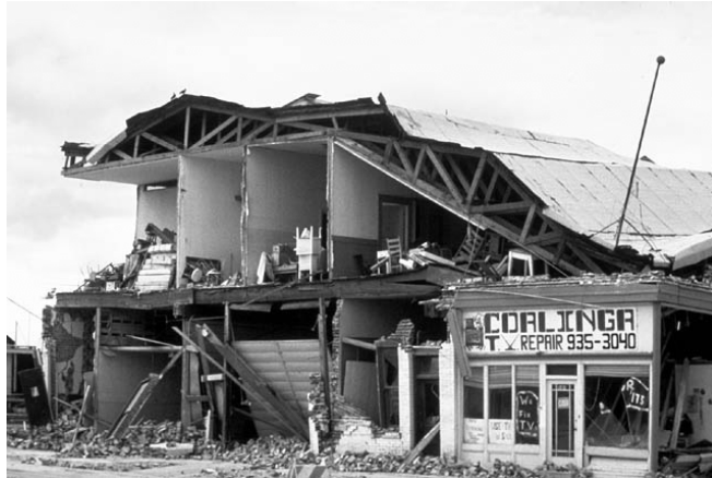
Figure 1. Out-of-plane wall failure in the 1983 Coalinga Earthquake.
