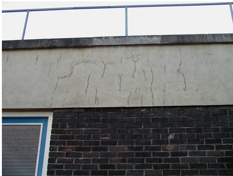
Figure 1. Typical shrinkage cracking of render.
