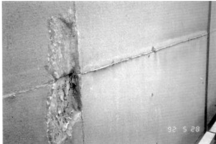
Fig 3 Stone panels spalling at compression joint due to excessive compression
