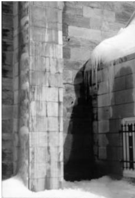
Fig 4 Buttress in 1997 Note ice formation at joints on left
