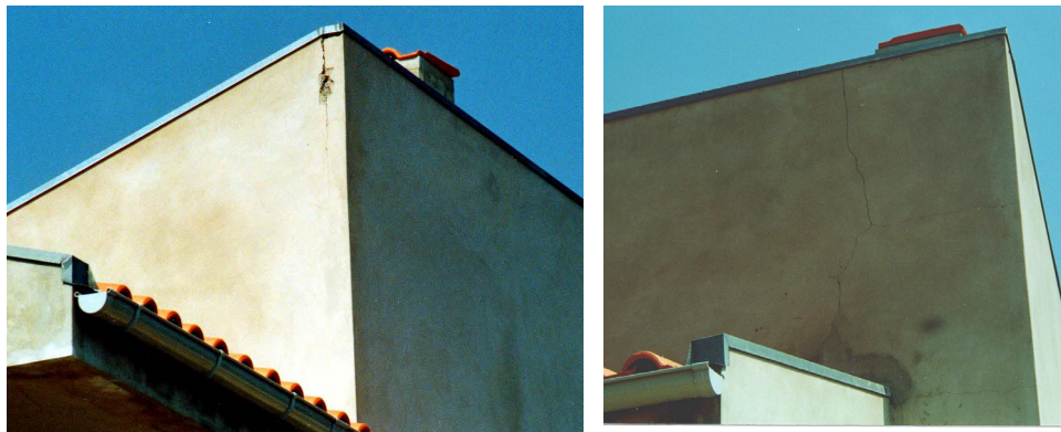
Figure 12. Cracking problems in the cottage complex.
