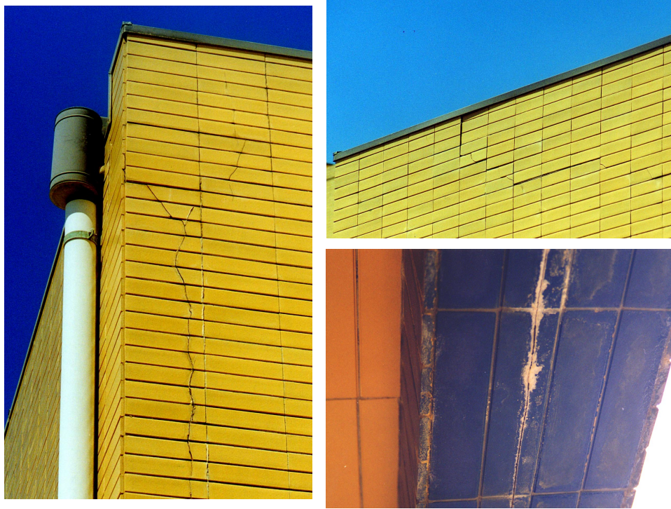
Figure 4. Hotel's cracking problems.
