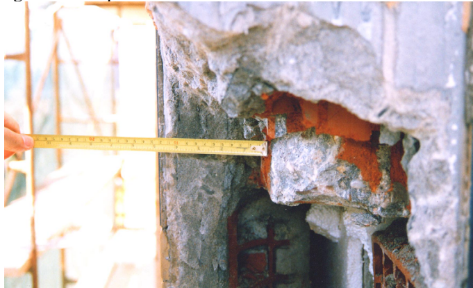
Figure 8. Prospecting carried out at the hotel to confirm the composition of exterior walls.
