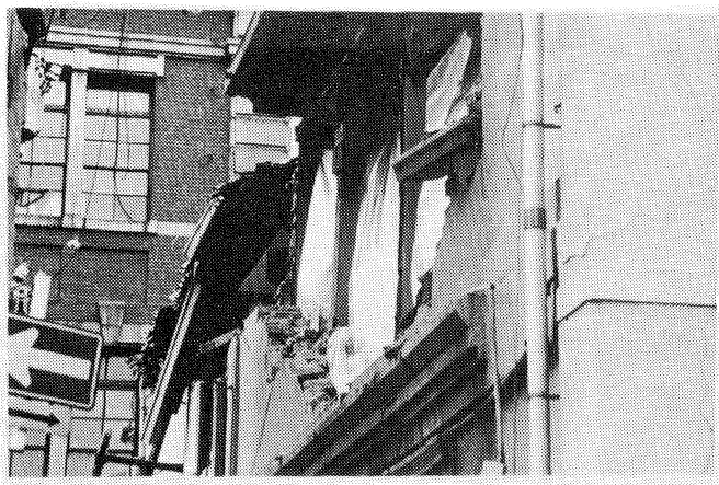
Figure 3c: Close-up view of out-of-plane damage to an unreinforced masonry building in downtown Kobe
