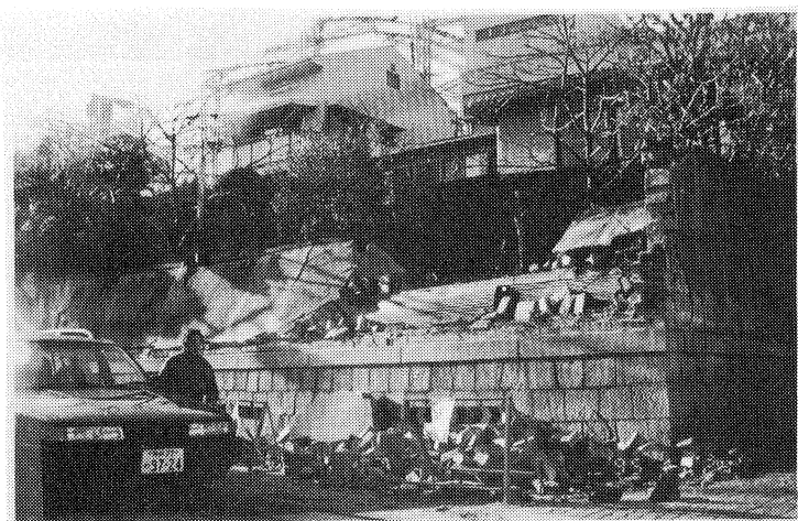
Figure 6b: Collapsed thick unreinforced masonry property wall
