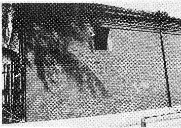
Figure 1d: Wall with visible in-plane cracking from an uncollapsed building of a sake-distillery complex
