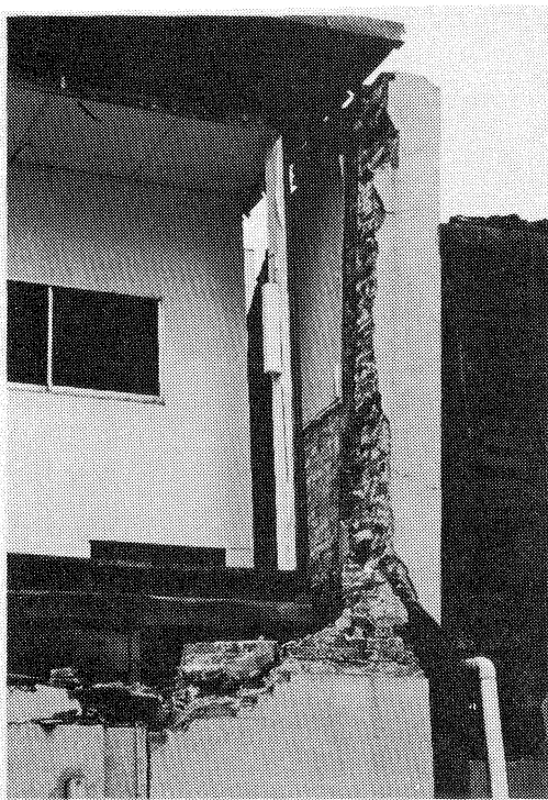
Figure 3d: Additional close-up view of out-of-plane damage to an unreinforced masonry building in downtown Kobe
