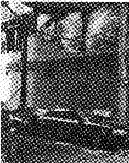
Figure 3b: Additional global view of out-of-plane damage to an unreinforced masonry building in downtown Kobe
