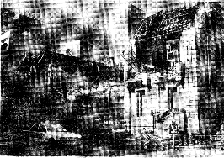
Figure 2a: Severely damage unreinforced masonry building in Downtown Kobe (global view)
