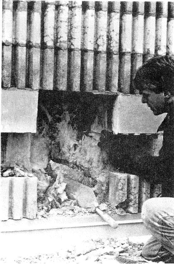
Photo 12 - Air Leakage from Top of Flashing
