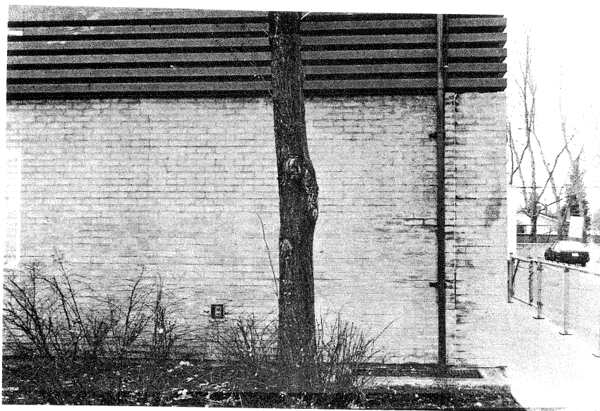
Photo 2 - Saturated Brick on Administration Wing
