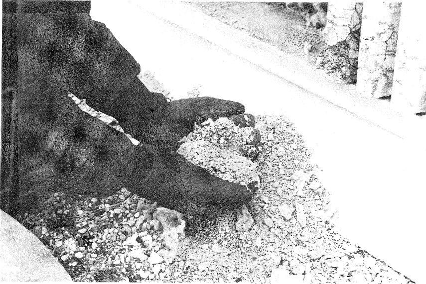
Photo 11 - Serious Concrete Block Deterioration
