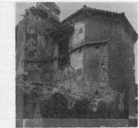
Fig. 2 - Church of S.Maria di Fossale (Friuli) damaged by the earthquake of 1976.
