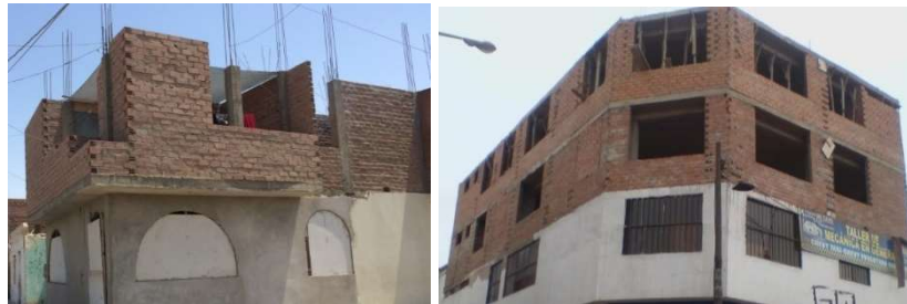
Figure 2: Popular informal buildings have walls made of horizontally-hollow bricks
