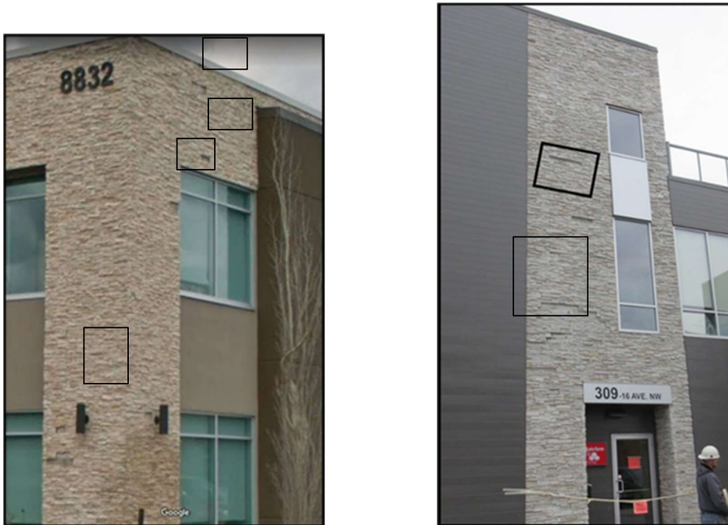
Figure 1: Bond failures in Adhered Thin Masonry Veneers [1]
