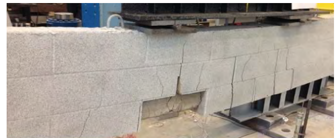
Figure 11: Failure mode of specimen F-6W
