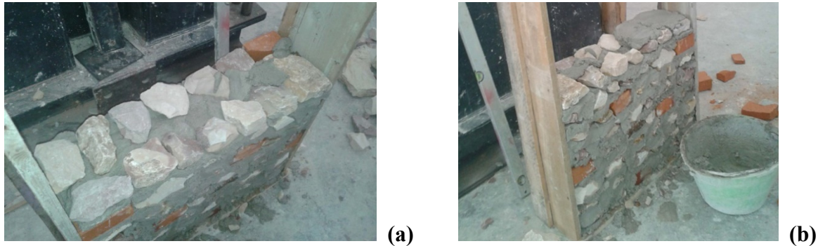
Figure 4: Wall Panels under Construction: (a) Detail of the Horizontal Cross Section; (b) Lateral View
