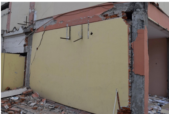
a) Cracking around infill panel perimeter
