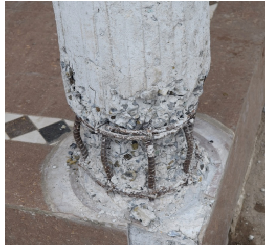
Figure 8: Column compression failure
