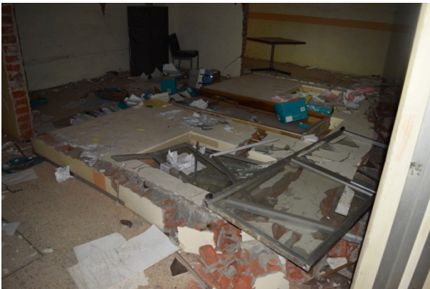
a) Collapsed interior URM partition
