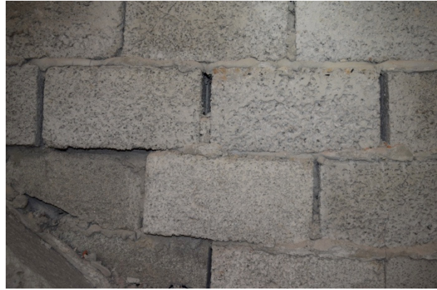
Figure 3: Open head joints
