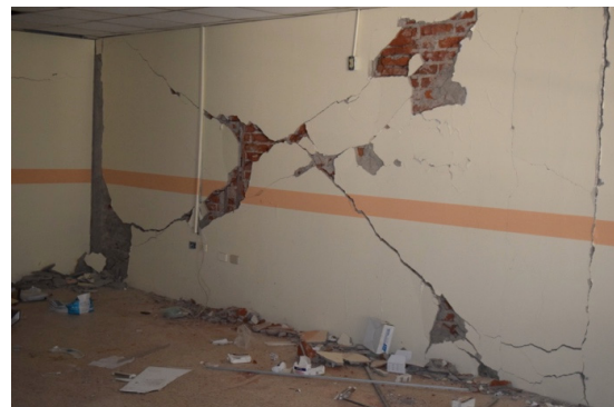
b) Bidirectional diagonal cracking
