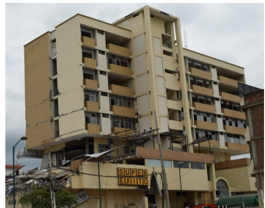
b) Discontinued RC infill frame
