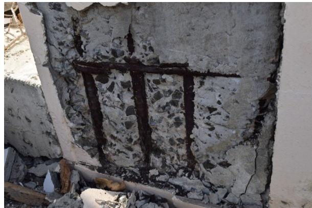
Figure 2: Corroded reinforcing bars
