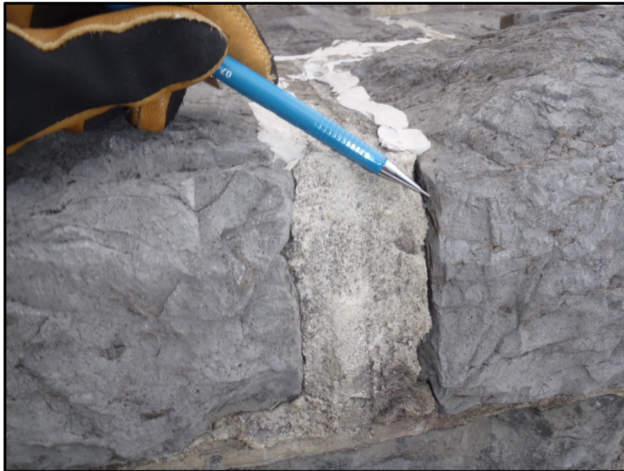
Figure 1: Cracked Mortar Joints
