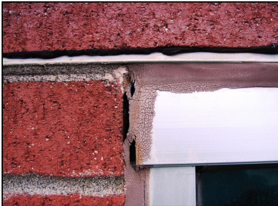
Figure 3: Failed Sealant Joints
