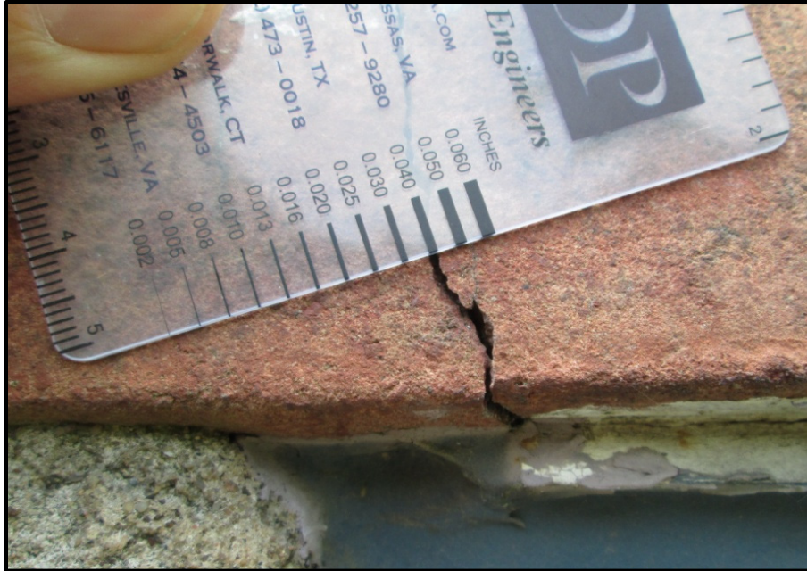
Figure 2: Cracked Masonry Units
