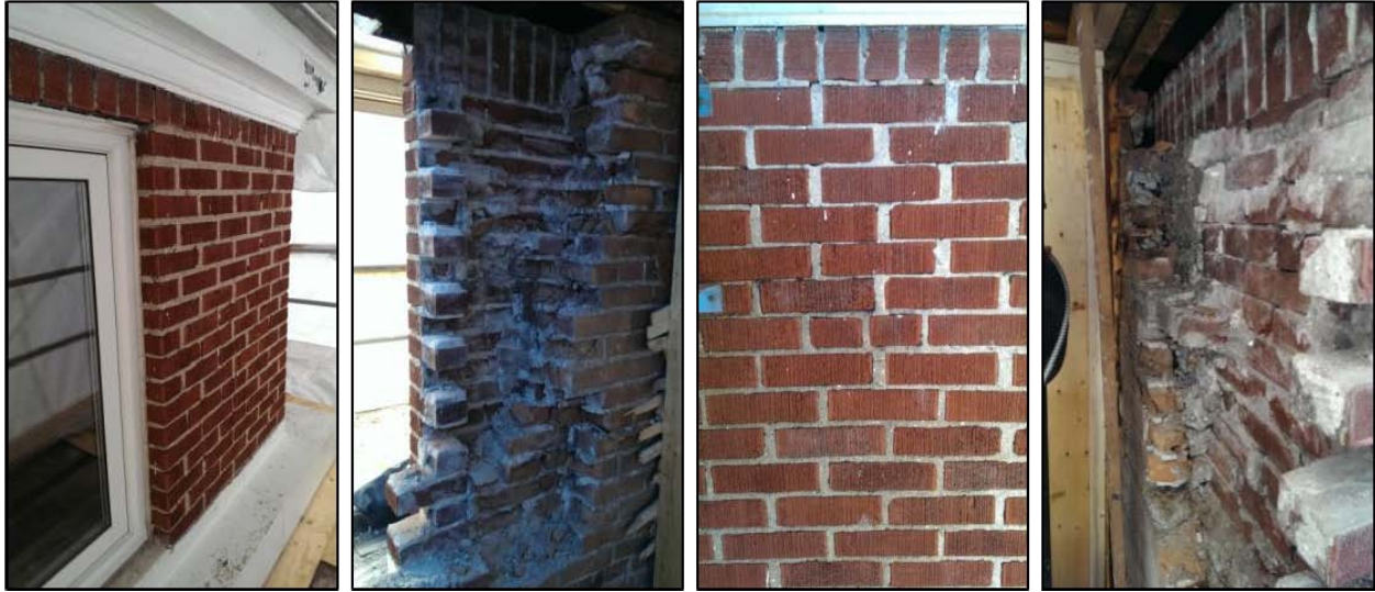
Figure 6: Condition of Masonry Wall as Observed on November 7, 2013
