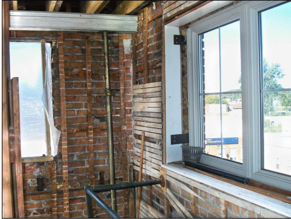
Figure 4: Brick Deterioration (September 17, 2013)
