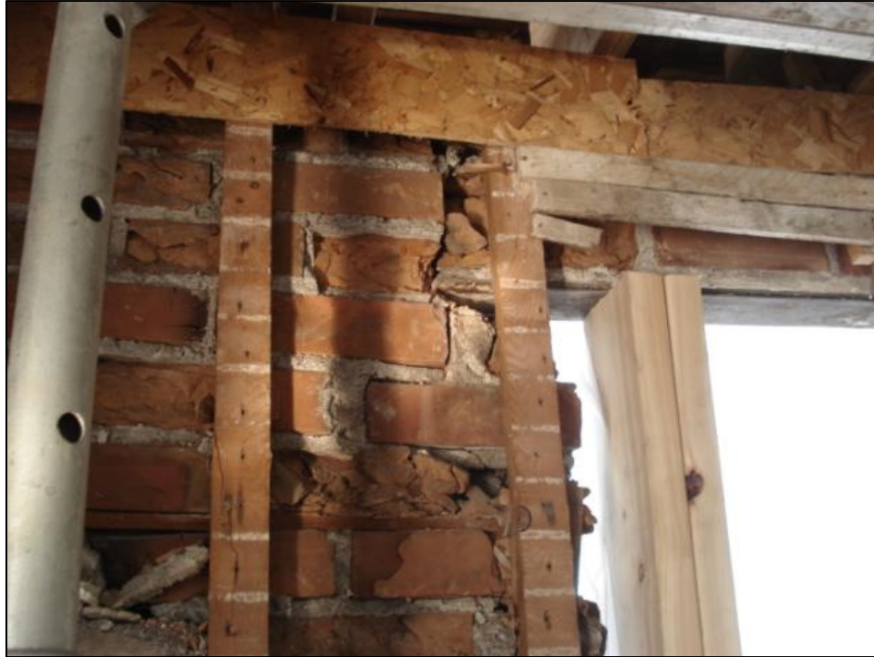
Figure 3: Severe Brick Deterioration (August 19, 2013)
