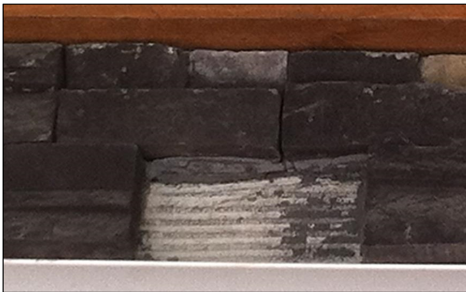
Figure 2: Failure Mode II - Bond Failure at the Scratch coat/Setting bed interface (scratch coat visible).
