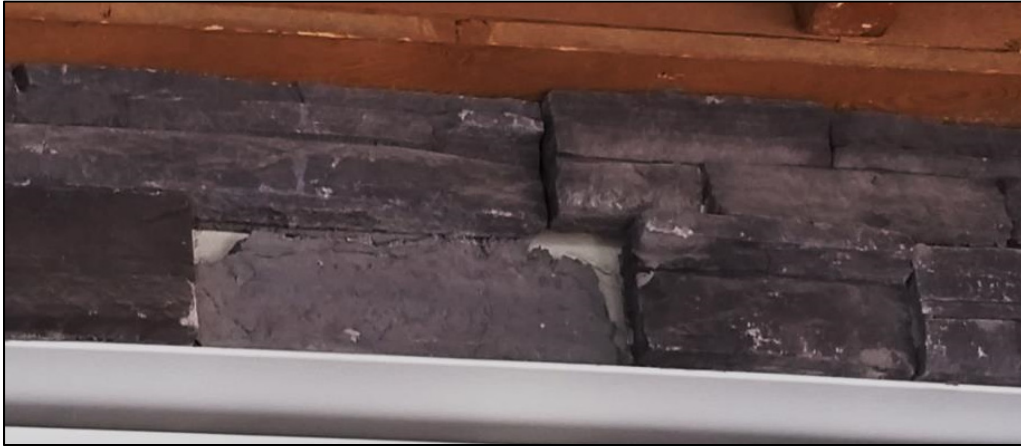
Figure 1: Failure Mode I - Bond Failure at the Stone Unit/Setting bed interface (setting bed visible).
