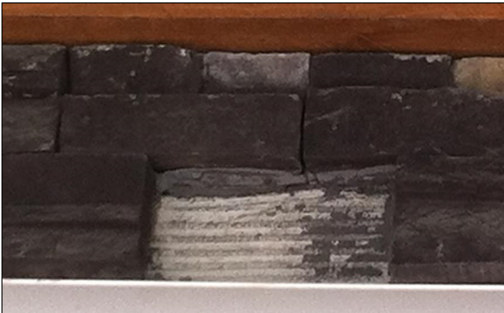
Figure 3: Failure Mode II- Bond Failure at the Setting Bed Mortar/Scratch coat interface (scratch coat visible) – photograph courtesy of Alberta Masonry Council.
