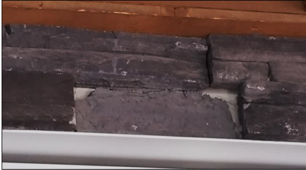
Figure 2: Failure Mode I - Bond Failure at the Setting Bed/Stone Unit interface (setting bed mortar visible) – photograph courtesy of Alberta Masonry Council.
