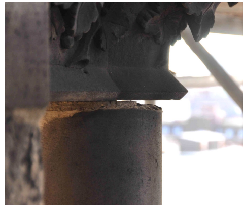
Figure 7: Mortar Erosion at the St. Nikolai Memorial
