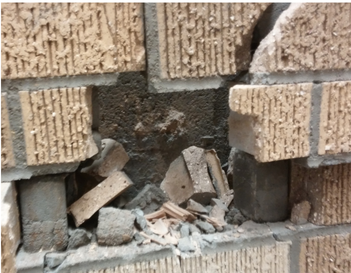
Figure 13: Front face of CMU Wall on Modular Brick Veneer Specimen 2 Behind Missile
