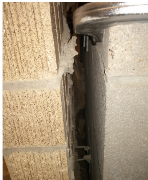
Figure 8: Brick Pieces Pushed Against the Block Face on the Utility Unit Specimen 1
