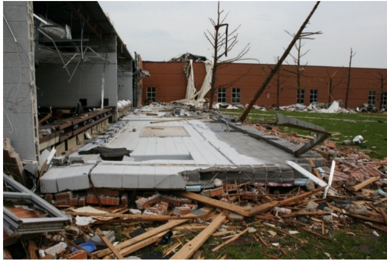
Figure 1: Tornado Wind Damage of a School in Joplin MO
