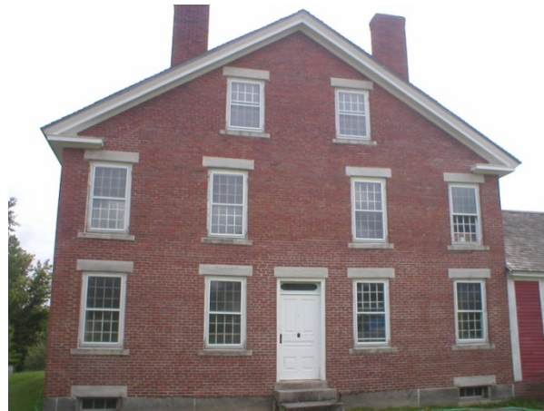
Figure 6: 1848 Tavern with Deflection, Bowing and Cracking around Door
