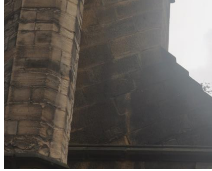
Figure 11: The Buttress with Inclined Stone Blocks Added to Prevent the Out-of-Plane Mechanism of the South Wall
