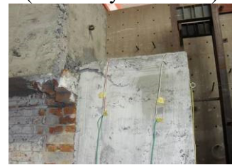
(f) Failure on Top of Concrete Wall (Interstory drift 1/100)
