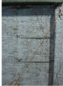
(b) Crack of Masonry Wall (Interstory drift 1/50)
