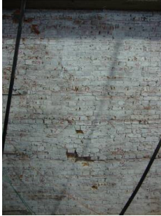
(a) Brick Fracture (out-of-plane distortion) (Interstory drift 1/50)
