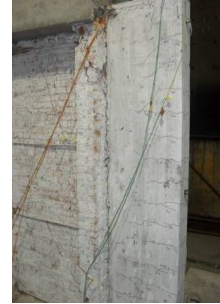
(c) Crack of Concrete Wall (Interstory drift 1/50)
