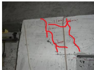
(b) Crack of Concrete Wall 1
