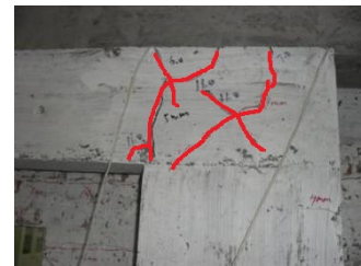
(c) Crack of Concrete Wall 2
