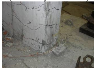
(e) Failure on Bottom of Concrete Wall (Interstory drift 1/50)
