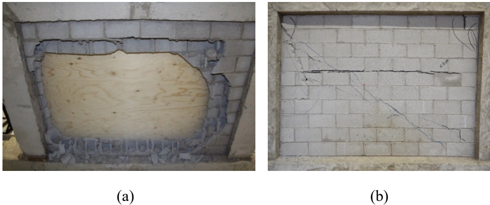
Figure 4: (a) Out-of-Plane Failure Mode of IF-ND, (b) In-plane Failure Mode of IF-D2
