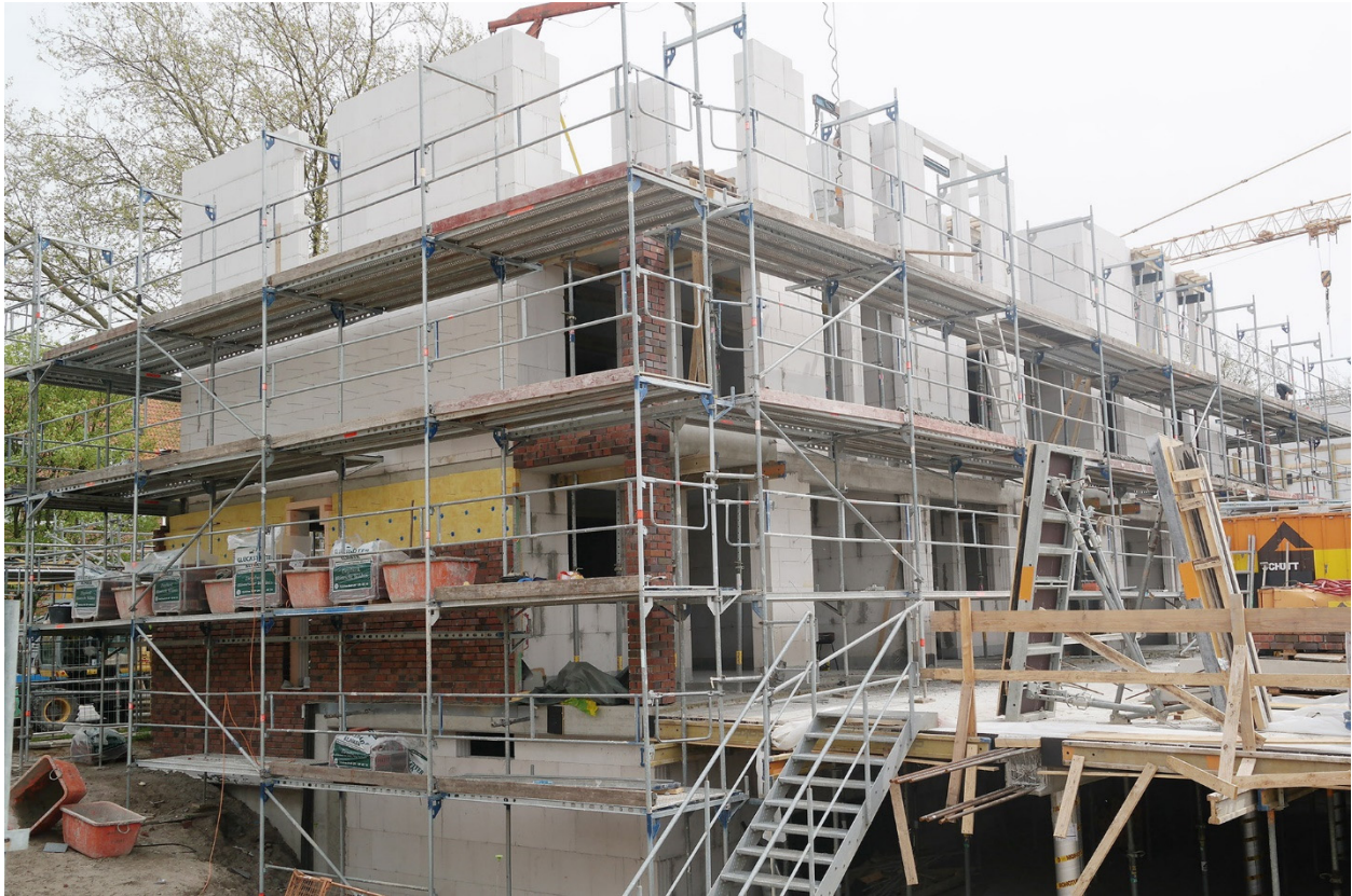
Figure 1: Construction of masonry veneer walls in northern Germany according to Eurocode 6: Backing walls are made of calcium silicate blocks with thermal insulation (mineral wool) and masonry veneer of brickwork
