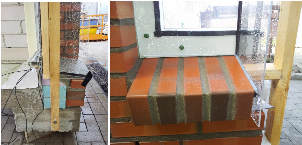
Figure 8: Test walls with masonry veneer and window surface after lab rain exposure [4] Left: Sill plate and installed humidity sensors. Right: Brick sill.
