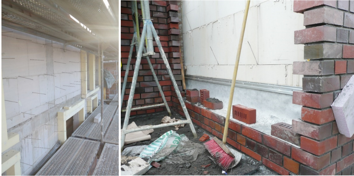
Figure 5: Left: Backing wall (calcium silicate-blocks) with anchorage and bars of extruded polystyrene foam (XPS), framing openings for floor level window to minimize heat loss. Right: Flashing for waterproofing at the footing of the cavity of a masonry veneer wall (sheets of welded polymerized bitumen). Because the sheets have to be manually resealed around edges, the water tightness at corner sections is critical.
