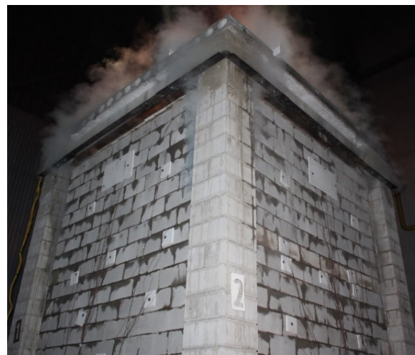
Figure 3b: Moisture bleeding off of the walls
