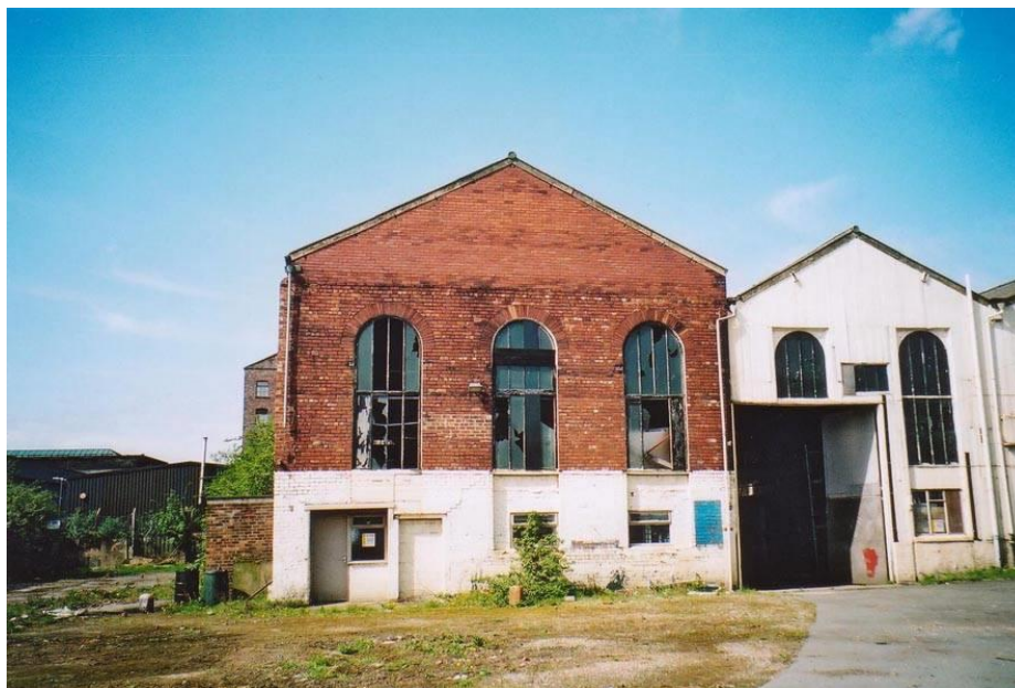
Figure 2: The Machine Shop
