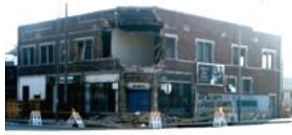
Figure 6: Typical Corner Damage
