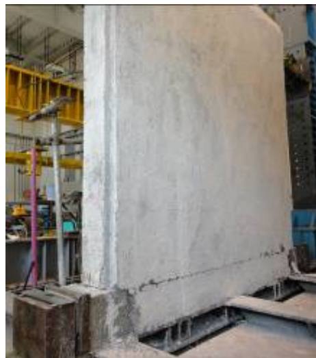
Figure 12: Rocking Failure Mode of Retrofitted Wall with Shotcrete Layer
