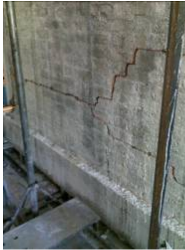
Figure 6: Crack Pattern of Traditional URM Wall under Cyclic Loading
