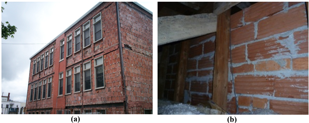
Figure 1: (a) School building with structural clay tile infilled steel frames; (b) Structural clay infills in roof space of typical school building.
