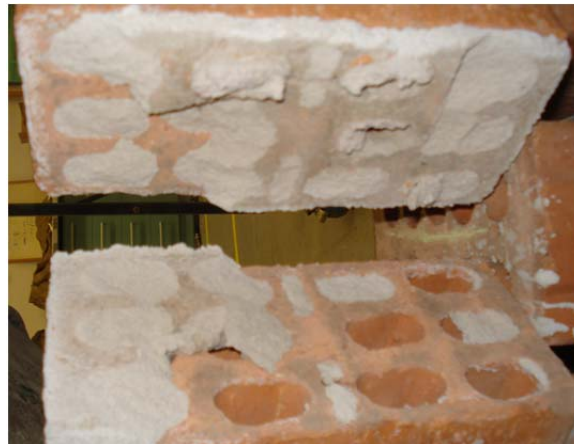
Figure 9: Typical failure mode for triplet tests. Note: the penetration of mortar into the cores was greater onto lower bricks (bottom of joints); however there was no trend observed with regard to which surface actually failed in shear (roughly half for each surface)
