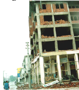
(d) Infill Failure due to Out-of-Plane Loads
