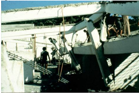
(a) Failure of Beam-Column Connection
