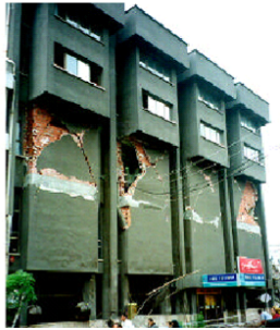
(c) Infill failure due to In-Plane loads
