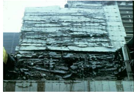
(b) Punching Shear Failure of Flat Plate
