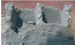
(a) Compression failure of blocks
