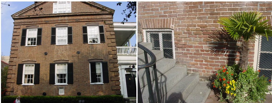
Figure 5: Buildings on Glebe Street on the College of Charleston campus: left) 20 Glebe Street, showing typical post-event “earthquake bolt” (pattress plate) repair; right) close up of 12 Glebe Street showing mortar deterioration due to moisture migration through the wall.
