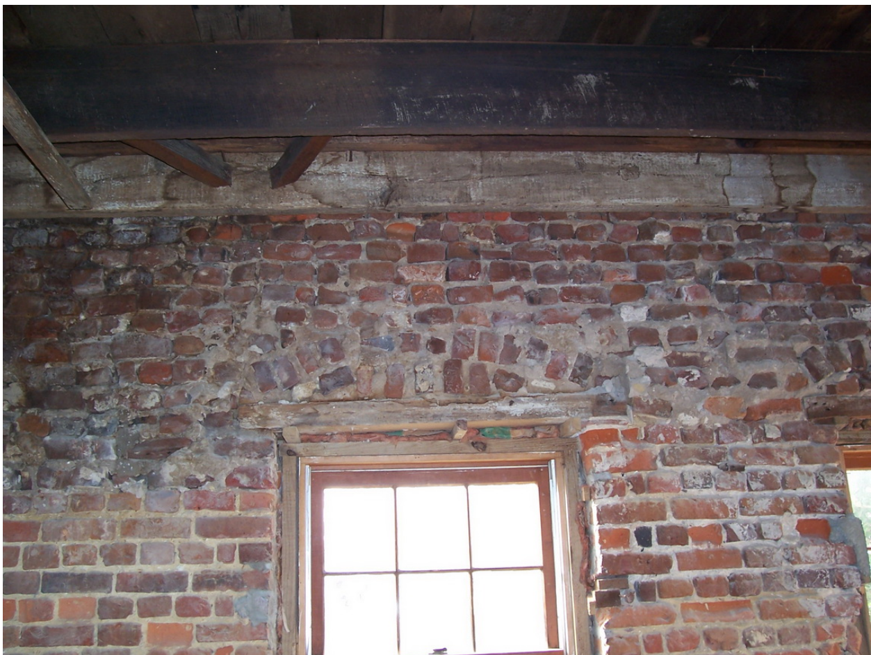
Figure 4: Interior view of the top (third) floor of an unreinforced masonry wall, originally built in 1785. Lower quality construction in the upper portion is the 1886, post-earthquake, reconstruction.
