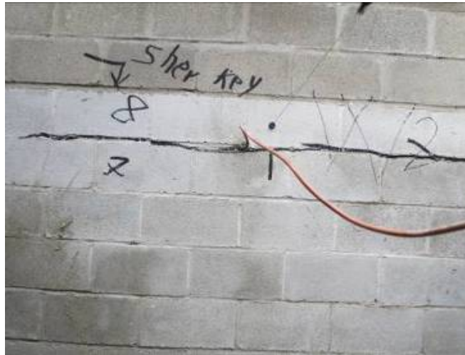
Fig. 6: Tension crack pattern of first masonry specimen after the detonation of 5.0 kg Pentex-D charge
