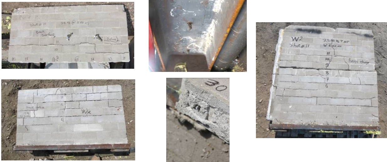
Fig. 8: Sample of compression spallings, tensions cracks, and bar fracture after the third shot
