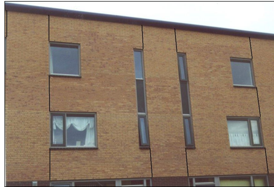
Figure 1: Many movement joints in a residential building
