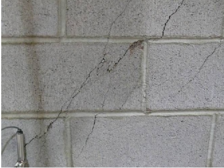
(a) Diagonal Cracking.
