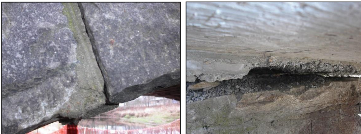
Figure 3: a) Opening in Mortar Joints between Exterior Ring Stones; b) Gap between Bottom of Northeast Spandrel Wall and Top of North Abutment
