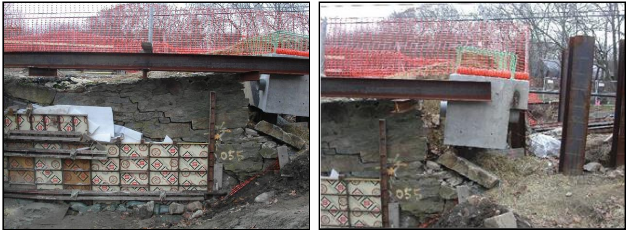
Figure 2: a) Failure of South Arch and Cracked Spandrel Wall; b) Rotation of New South Abutment
