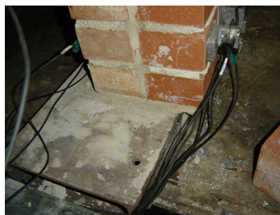
Figure 4: Sliding failure of CNT-I under the eccentric applied load
