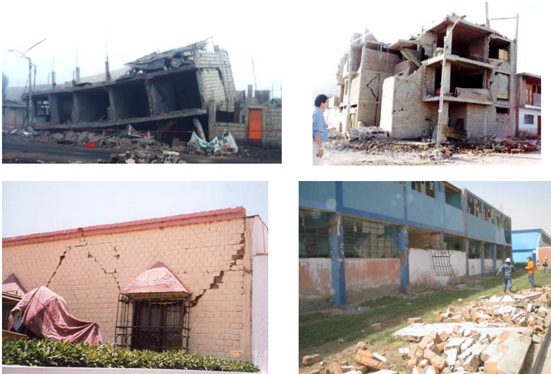
Figure 5: Damage to masonry constructions after the 2001 Atico (top) and the 2007 Pisco earthquakes (bottom)
