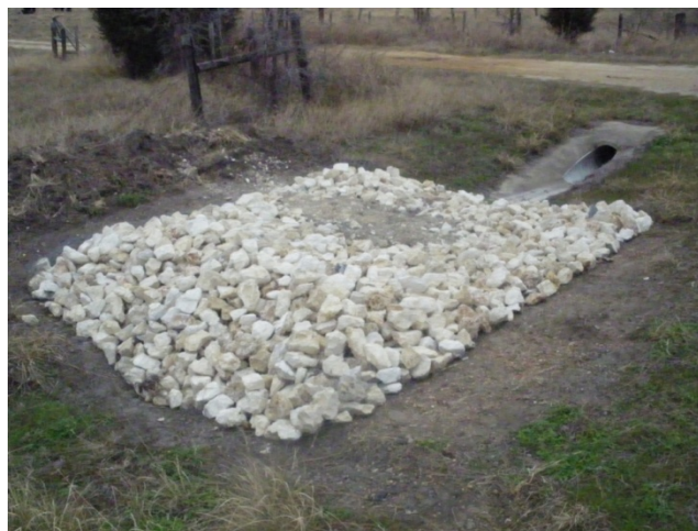
Figure 3: Simple TxDOT Sedimentation Trap
