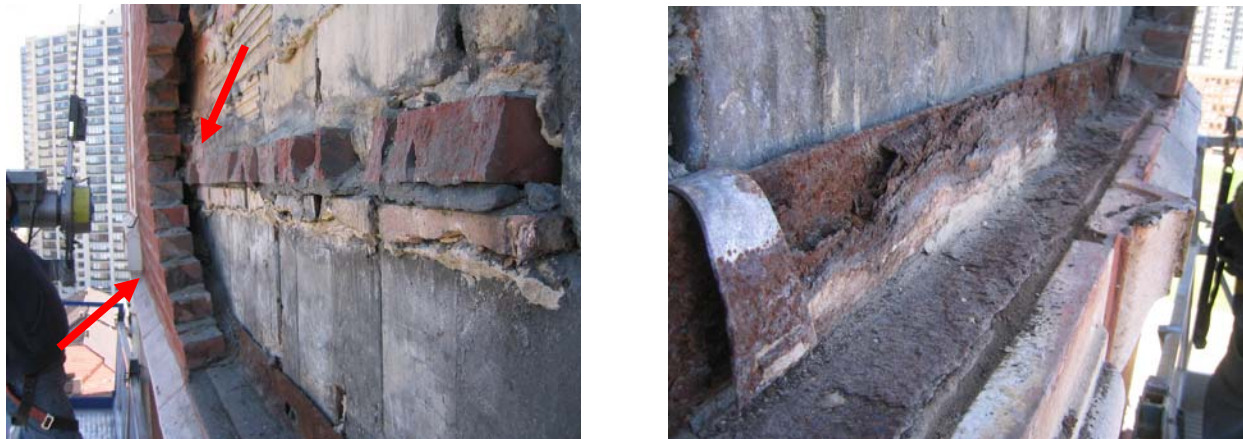
Figure 3: Representative examples of conditions found in Case Study 2: a) Cracked headers and displaced parapet wall; b) Significantly corroded angle.
