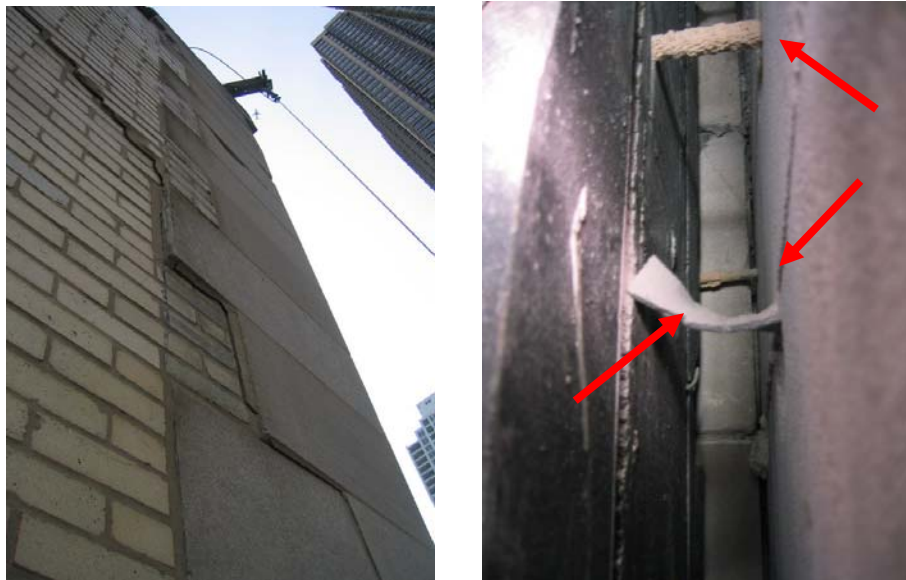
Figure 4: Representative examples of conditions found in Case Study 3: a) Displaced brick and limestone; b) Bent original dovetail anchor (left arrow) and new epoxy threaded rod stabilization anchors (right arrows).
