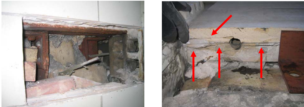
Figure 2: Representative examples of the conditions found in Case Study 1: a) Previous repair anchor remaining after removal of terra cotta unit; b) Shear cracks through terra cotta unit behind exterior face (note: angle on right side of photograph was installed as a temporary support).
