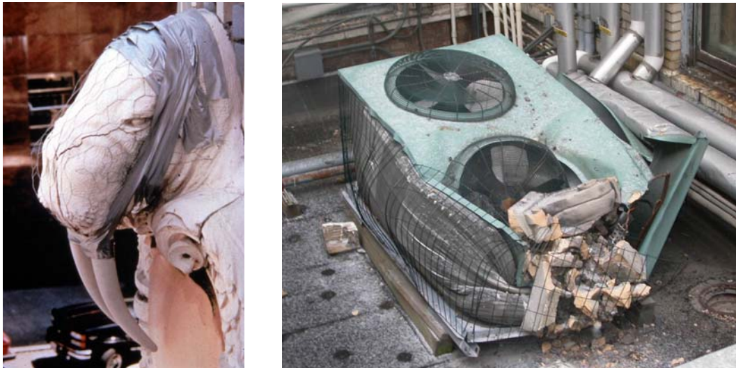
Figure 1: Examples of inappropriate maintenances resulting in public safety conditions.
