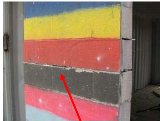
Damaged mortar joint at mid-height
