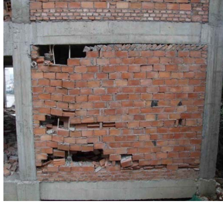
Figure 1: Infill damage after the 2008 Wenchuan, China earthquake [1]
