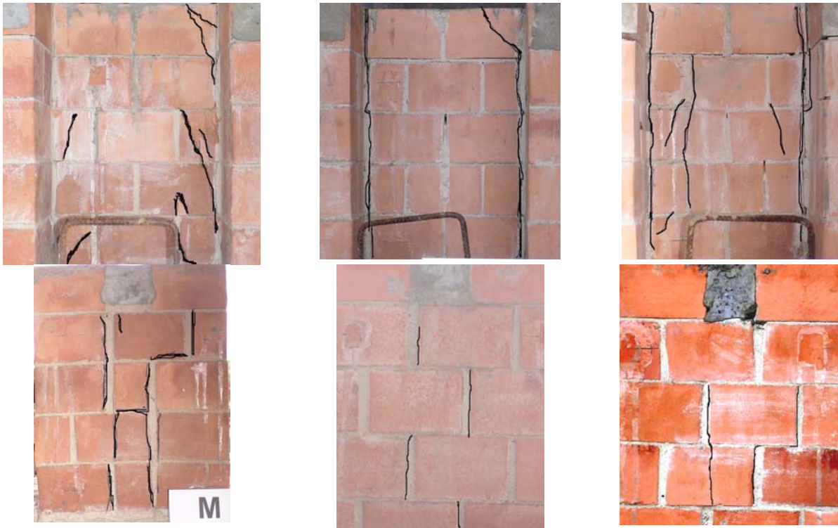
Figure 4: Comparison of typical failure patterns: a) Running bond (RB); b) Stack bond connected by steel trusses (SBT); c) Stack bond connected by steel U-staples (SBS)
