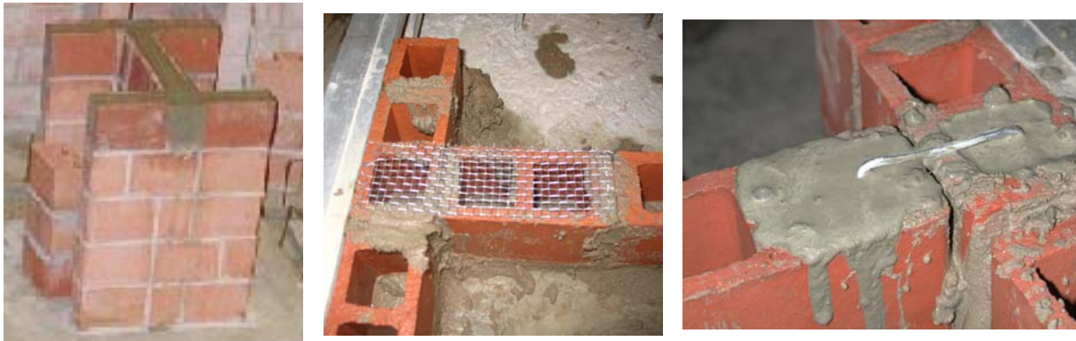
Figure 3: Vertical interfaces: a) Running bond (RB); b) Stack bond connected by steel trusses (SBT); c) Stack bond connected by steel U-staples (SBS)
